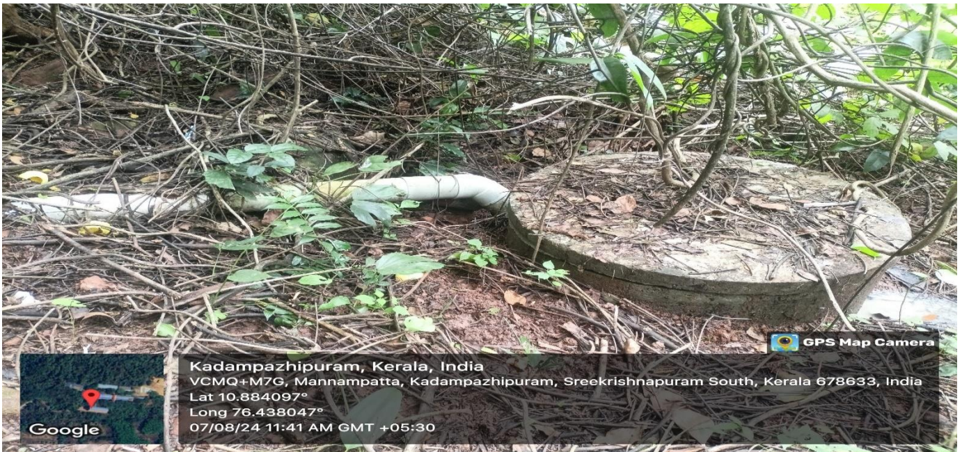
Sewage System in college
