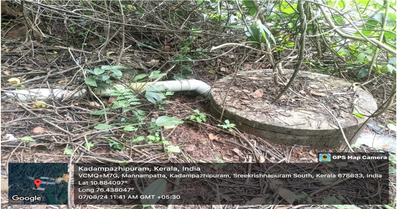
Sewage System in college
